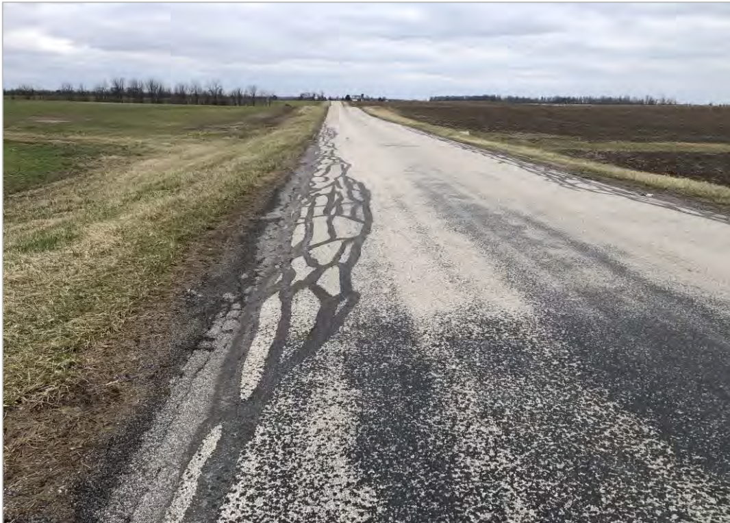
PHOTO 5: Distressed pavement (edge cracking) on CR22 near US 20, looking south.
